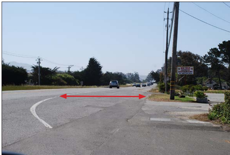
Top: Miramar looking north toward El Granada. Bottom: Miramar looking south. The photos show a lack of consistent built cross section width and characteristics and lack of defined inside and outside edges.
