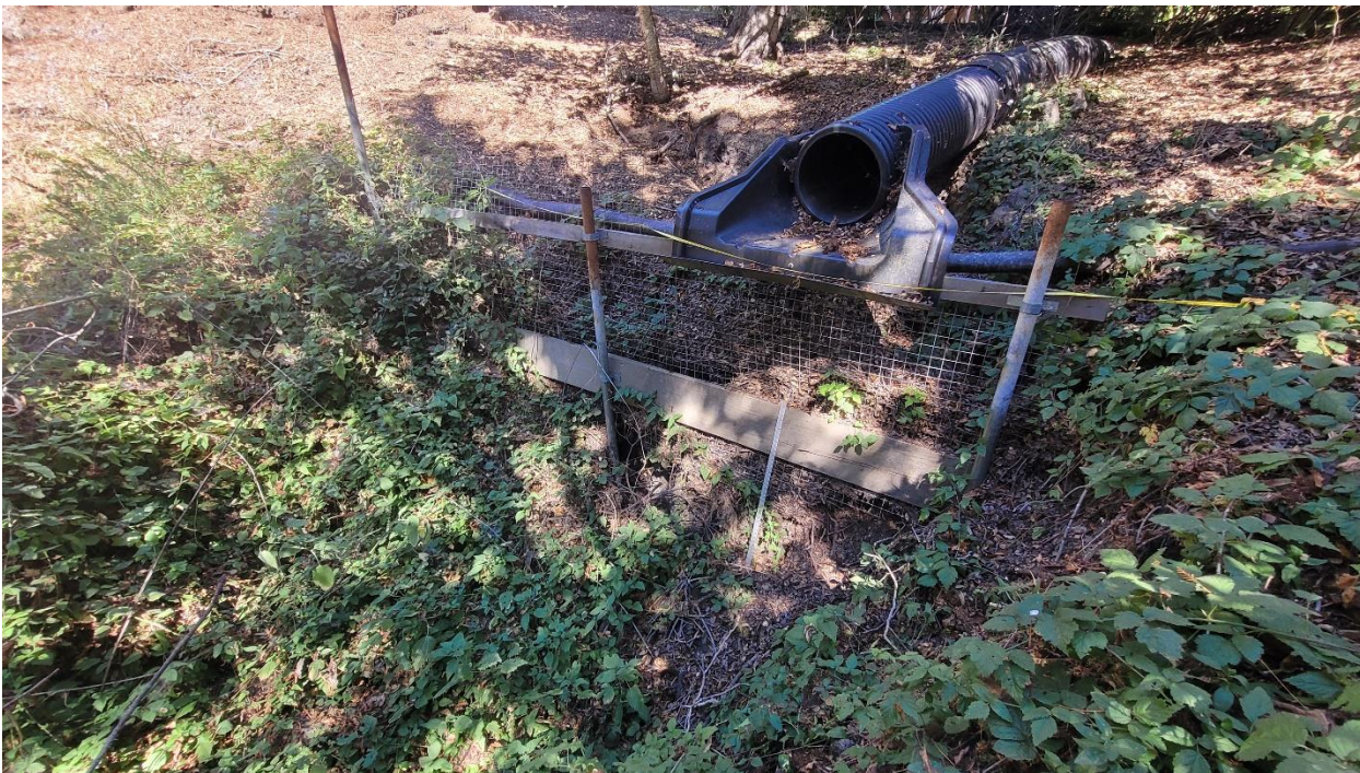
Photo 2: Erosion on parcel 078-120-060 from another culvert used to deliver runoff from the culvert in photo 1 around the wastewater drain field. Collapsed section measures approximately 18' long x 16' wide x 6' high. Stabilization fencing installed to slow erosion can be seen in the photo.
