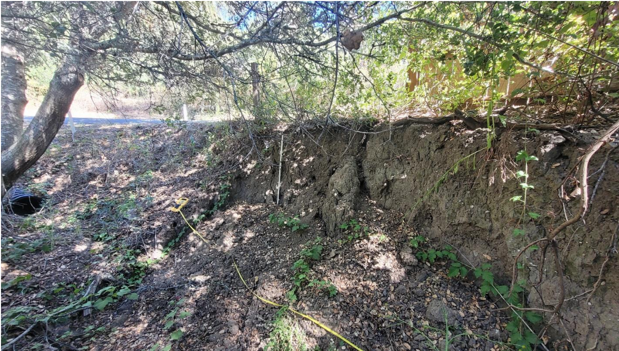
Photo 1: Soil destabilization within 3 ft of Old La Honda Road bed from the culvert that drains north portion of parcel 078-120-050 under Old La Honda Road. Collapsed section measures approximately 15' long x 3' wide x 3' high
