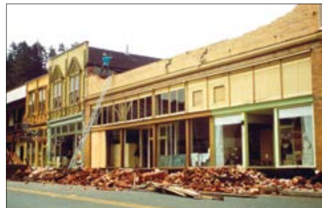
Bricks from the same building fell during the April 1992 earthquake. The building has now been replaced by a wooden structure.
